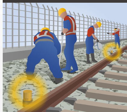
Authorized personnel's safety is ensured by a flashing beacon
