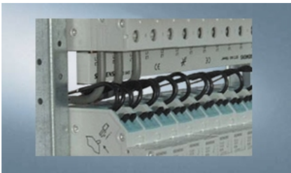
Plenty of space for wiring Clear overview and easy access to all lines
