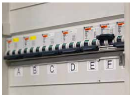
Circuit breaker marking
