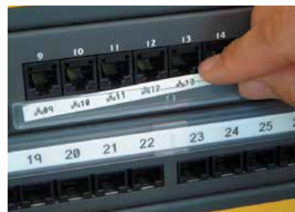
Punch block & patch panel labels
