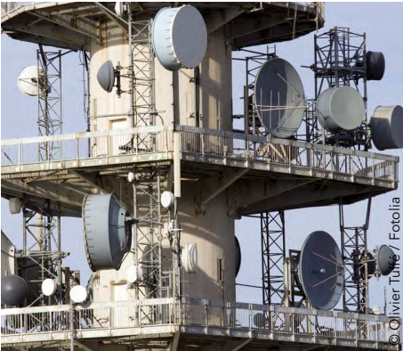
Telecom - Data infrastructure
