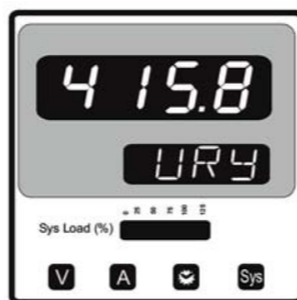
Screen 4 : Line to Line Voltage (Voltage between R and Y phase)
