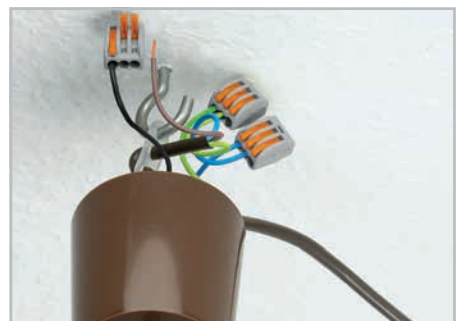
Lighting fixture connected with flexible power feed.
