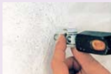
Strike conduit support
