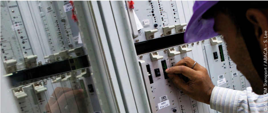
Railway - Closed from electrical operating areas
