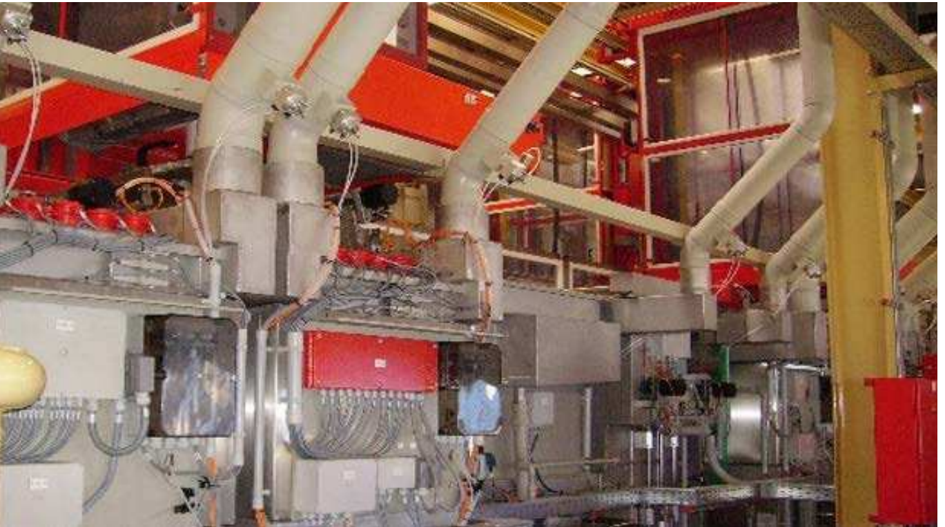
Chemical treatment plant at SKF
