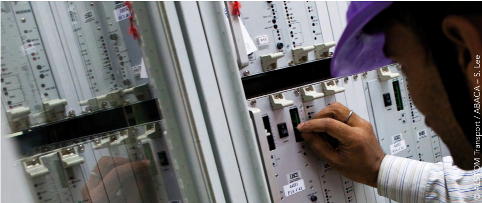
Railway - Closed from electrical operating areas
