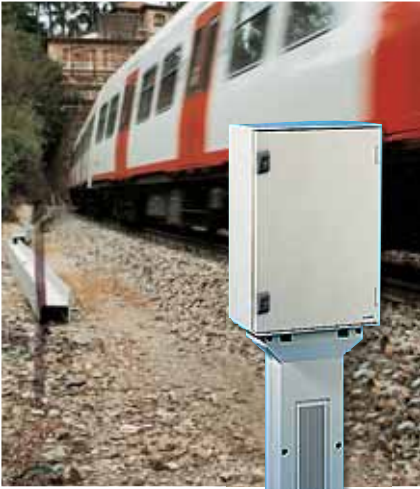
Outdoor installation, with exposure to atmospheric conditions: mist, solar radiation, extreme temperatures, etc.
