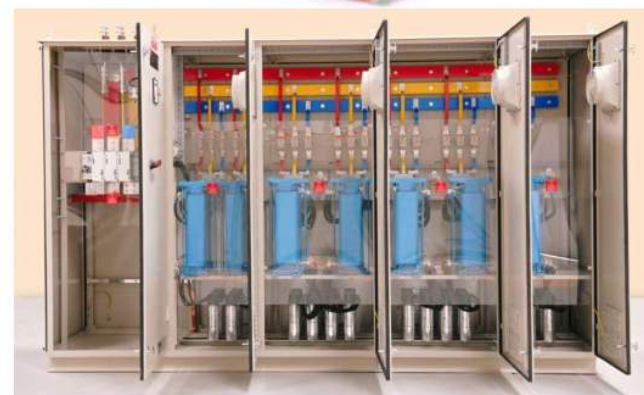
(de-) tuned Harmonic Filter
