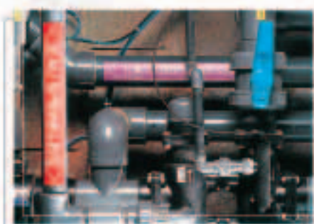
Identify pipelines on-site!
