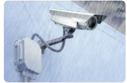
Installation with free cables
