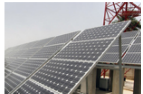
Solar-Powered Cellular Base Station
